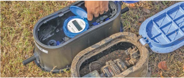
Pleased to 'meter' you: Introducing the new smart water meter (left), pictured here alongside the old-school, mechanical meter that is bowing out.
